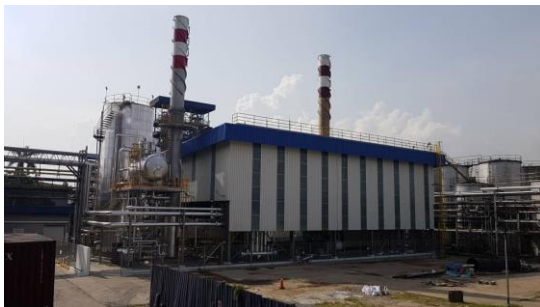
IOI Pan-Cen new combined heat and power cogeneration plant
