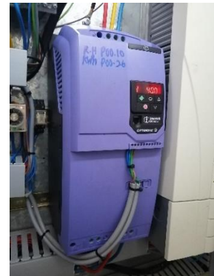
Newly installed Variable Speed Drive at IOIEO
