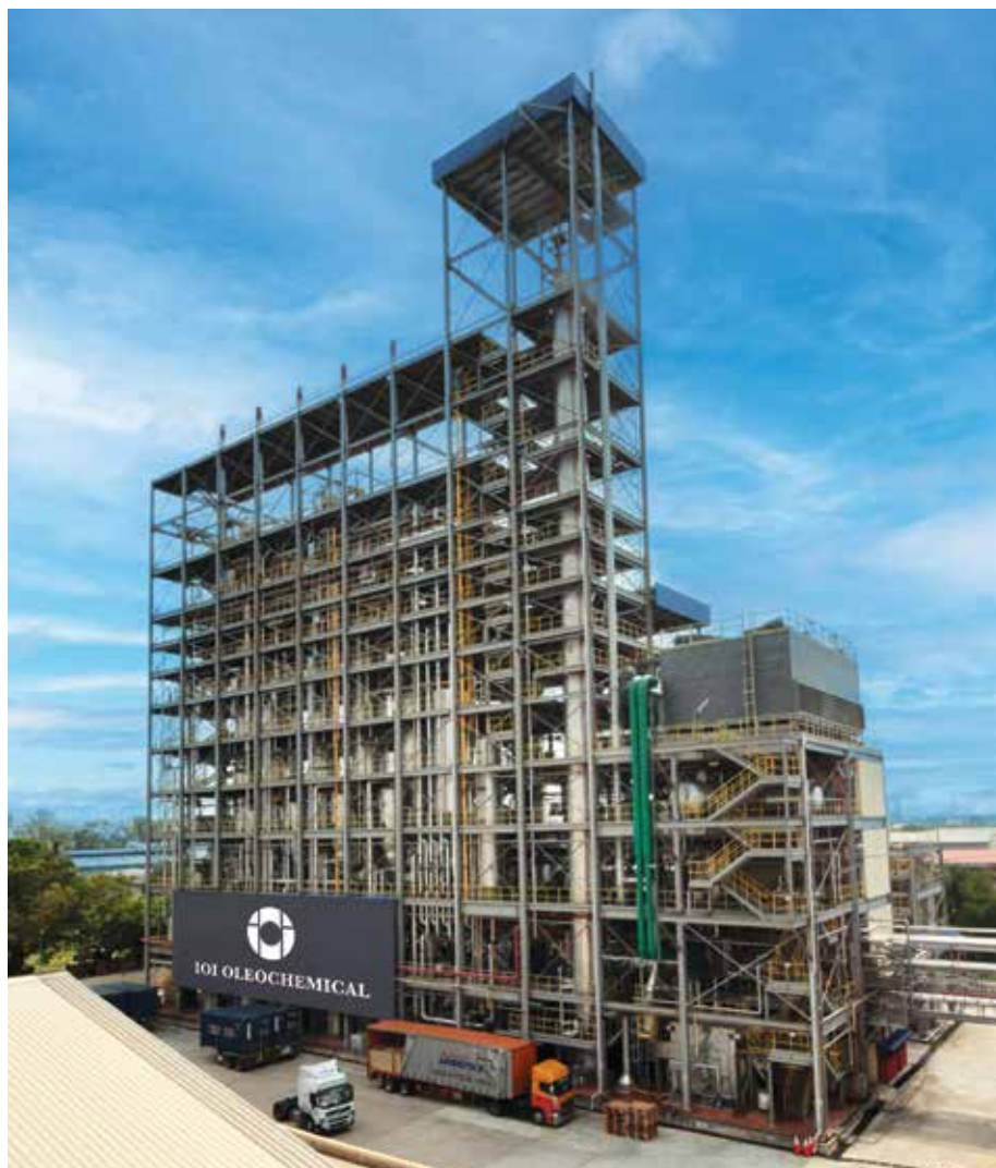
Our new oleochemical plant in Prai, Penang with a capacity of 110,000 MT per year.
